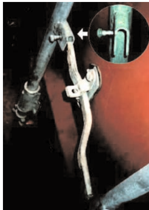
Figure 43.1: Main photo and inset show partly removed pin on sealed door handle.
