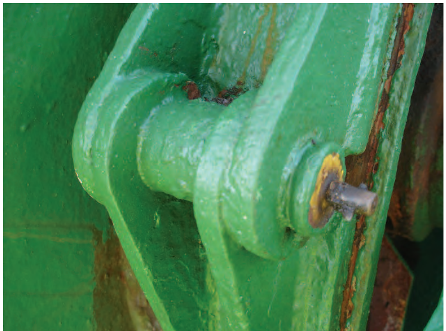
Ineffective grease point
