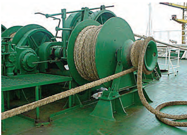
Well painted but poorly highlighted mooring station
